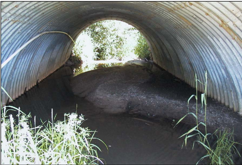
Figure 7.5 Temporary sediment storage in a culvert barrel, Little Bear Creek.
