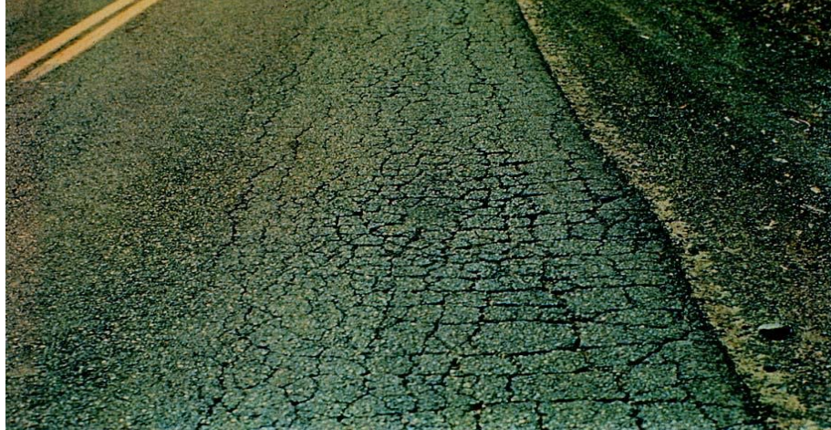
Figure 1.2 A Typical AC Pavement Fatigue Cracking
