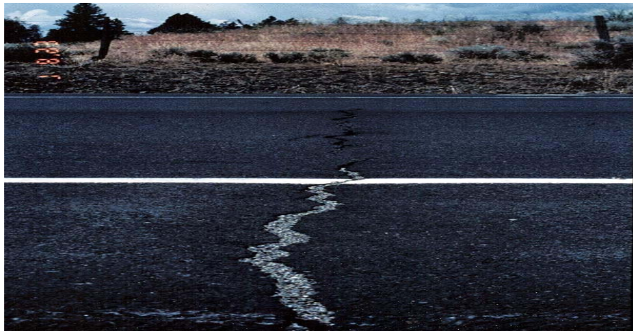
Figure 1.3 A Typical AC Pavement Thermal Cracking
