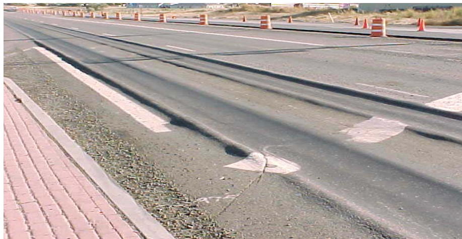
Figure 1.1 A Typical AC Pavement Rutting
