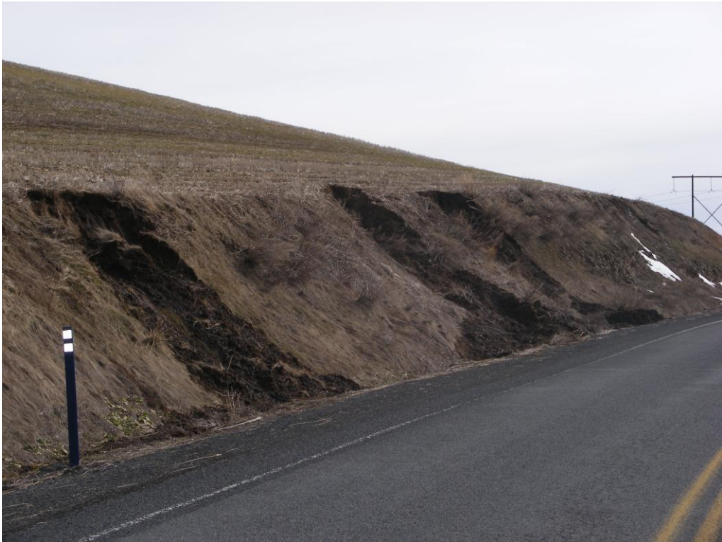
Photo 7: Hillside erosion east of Pullman, WA
