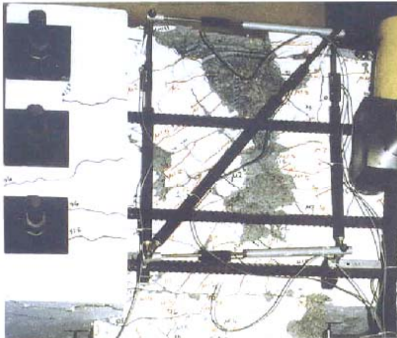
Figure 6.1 Crushing Failure Mode in a Knee Joint (Adapted from Sritharan and Ingham, 2003)
