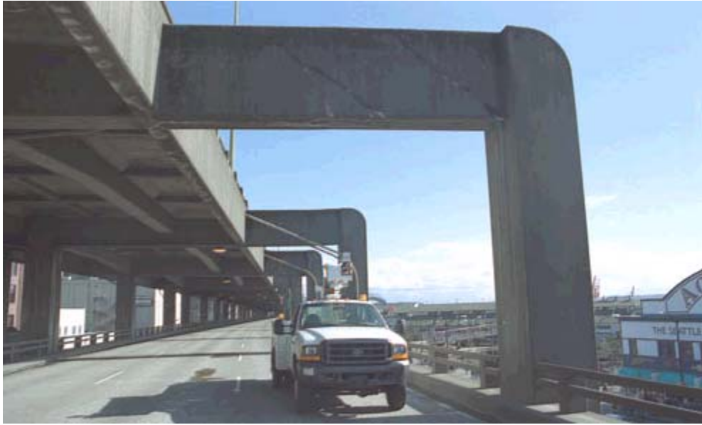
Figure 2.6 Cracking on Outrigger Beams, 2001 Nisqually Earthquake ( http://www.wsdot.wa.gov/projects/viaduct/deis/chapter1_1.htm )
