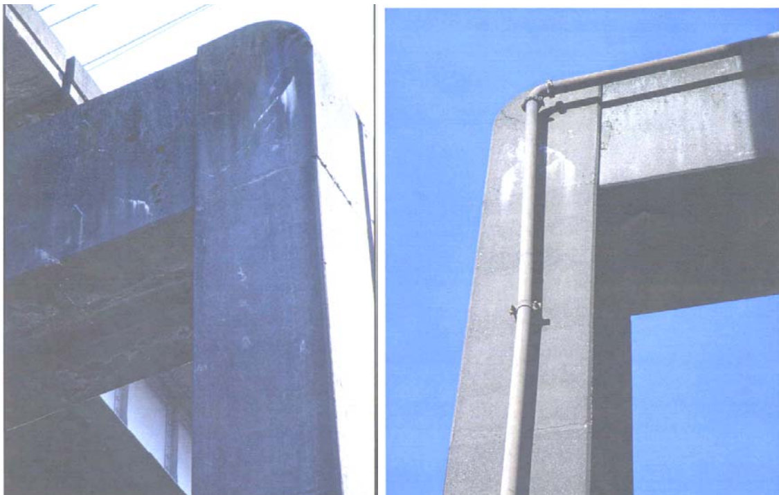
Figure 2.5 Cracks in Outrigger Knee Joints
