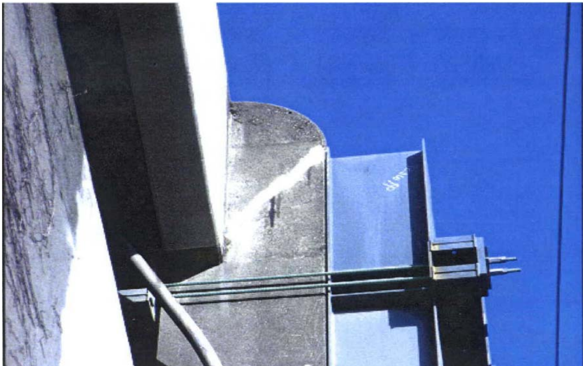
Figure 1.2 Damage to a Knee Joint in the Alaskan Way Viaduct
