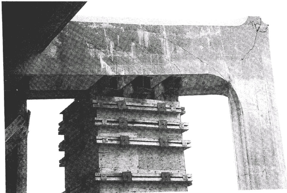
Figure 2.2 Damage to an Outrigger Bent in the I-280 China Basin Viaduct, 1989 Loma Prieta Earthquake (Adapted from Priestley et al., 1996)
