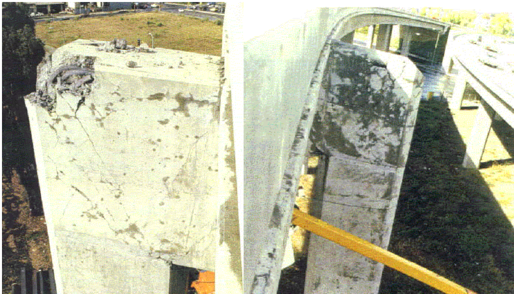
Figure 2.4 I-980 Joint Failure , 1989 Loma Prieta Earthquake (Adapted from Ingham et al., 1994a)
