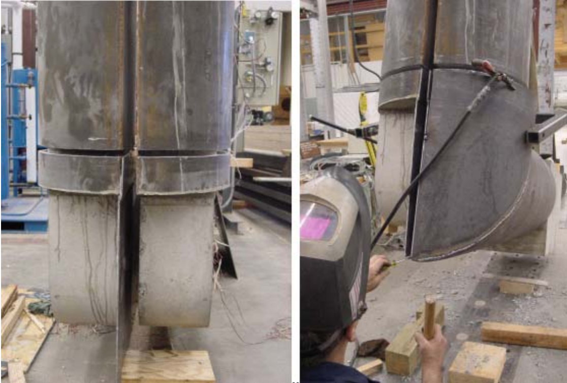
Figure 3.25 Retrofit Application Around the Beam and the Joint Showing the 3/4 in. (19 mm) New Gap, the Backside Plate and the Final Shape on One Side
