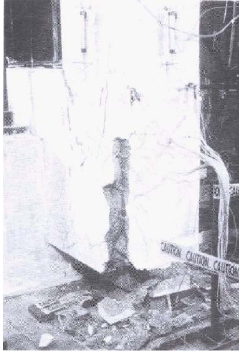
Figure 2.23 Bond Split Failure of the Knee Joint in the As-Built Short Specimen(Adapted from Stojadinovic and Thewalt, 1995)
