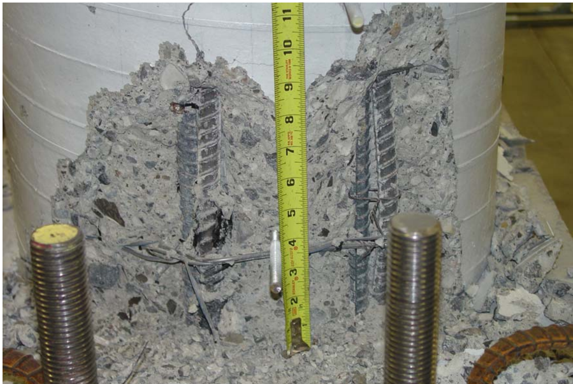
Figure 6.1-11 Spalling of the Concrete (Stapelton, 2004)
