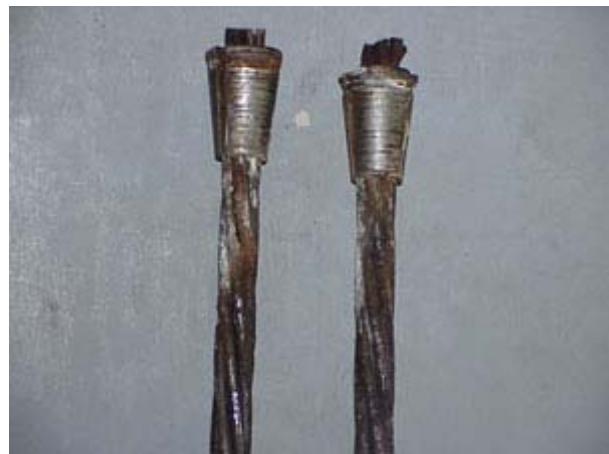
Figure 1.3 – Corroded strand ends removed from an anchorage in the Mid-Bay Bridge, Florida (Beitelman, 2000)
