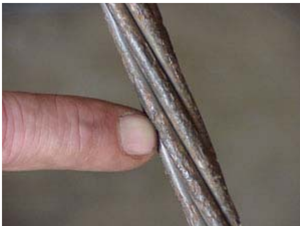
Figure 1.2 – Pitting corrosion on a post-tensioning strand from the Mid-Bay Bridge, Florida (Beitelman, 2000)
