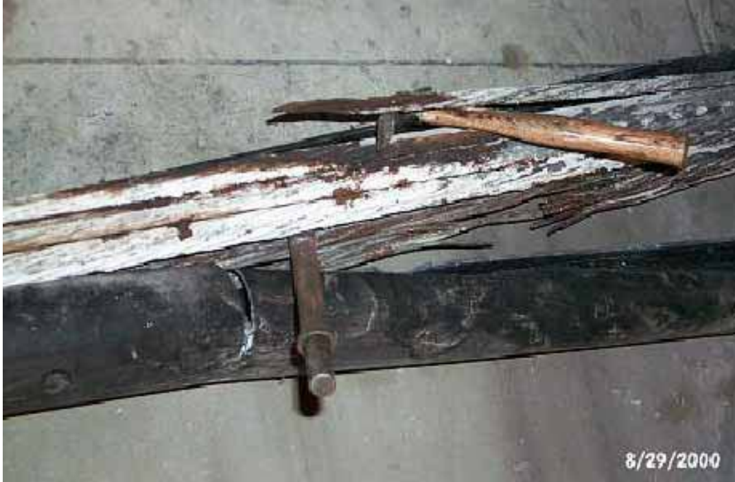
Figure 1.4 – Failure of a tendon in the Mid-Bay Bridge, Florida (Breen et al., 2004)
