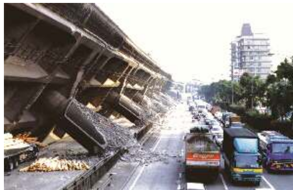
Figure 2.5.3: Collapsed of an 18-span viaduct section of Hanshin Expressway (from Ghasemi, 1996)
