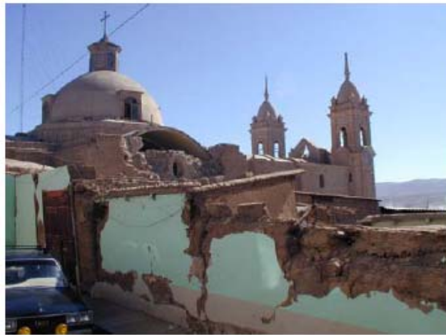
Figure 5.1.2: Cathedral in Moquegua, a stone structure with stone walls and stone vaults, sustained damage and lost one of its vaults (Photo by E. Fierro)
