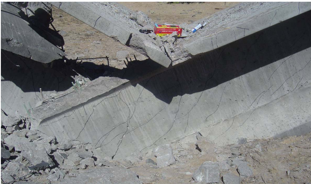
Figure 4-10: Damage from Blast Below, Experimental
