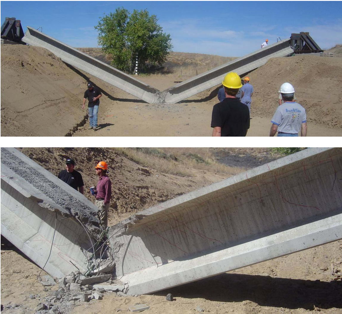
Figure 4-2: Damage from Blast Above, Experimental
