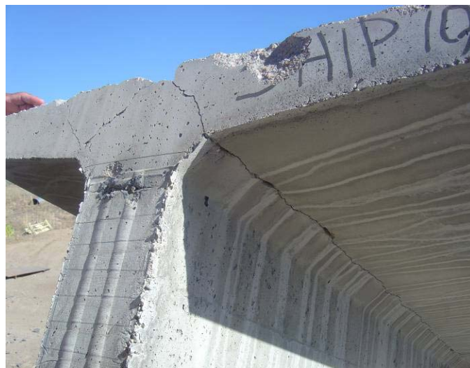
Figure 4-11: Longitudinal Cracking at Web-Flange Intersection
